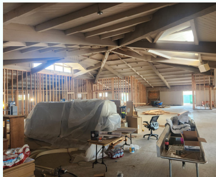
View of Hall from Kitchen Doorway New Walls going up—back left corner are the new restrooms
