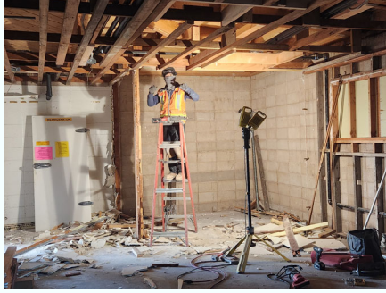
Walk in Refrigerator Demo
